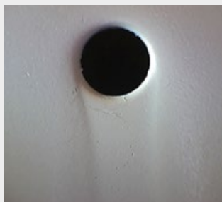
Strong sagging of paint
