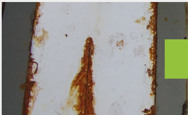
Weak corrosion protection in 2 layer system
